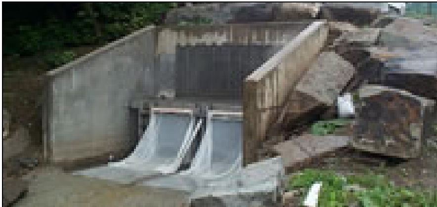
Fresh Creek Technologies Netting Trash Trap
